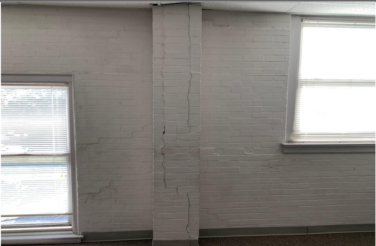
Deferred Maintenance – 4 th Floor
